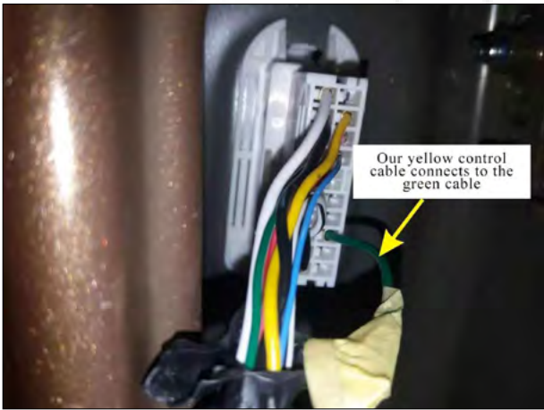
9. Central control cable connects the green cable.
